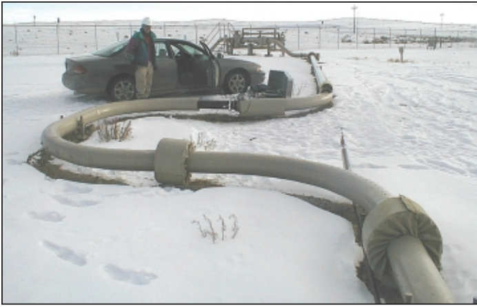
Figure 2 A short section of solid, straight 6-inch Inconel pipe approximately 12 inches long was found on this natural gas transmission pipeline to provide a site for the transducer installation.
